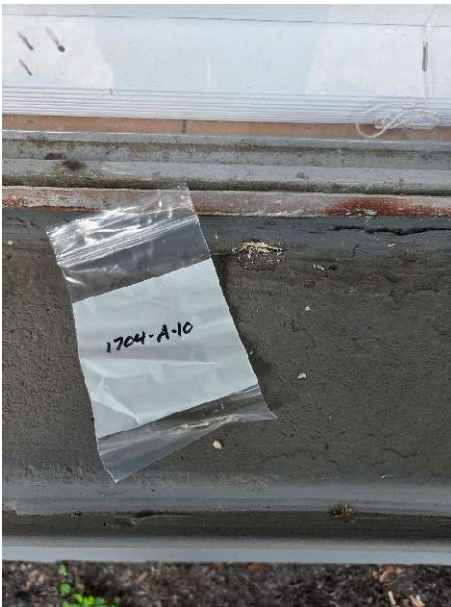
Sample 1704-10 Typical Exterior Caulking Sample
